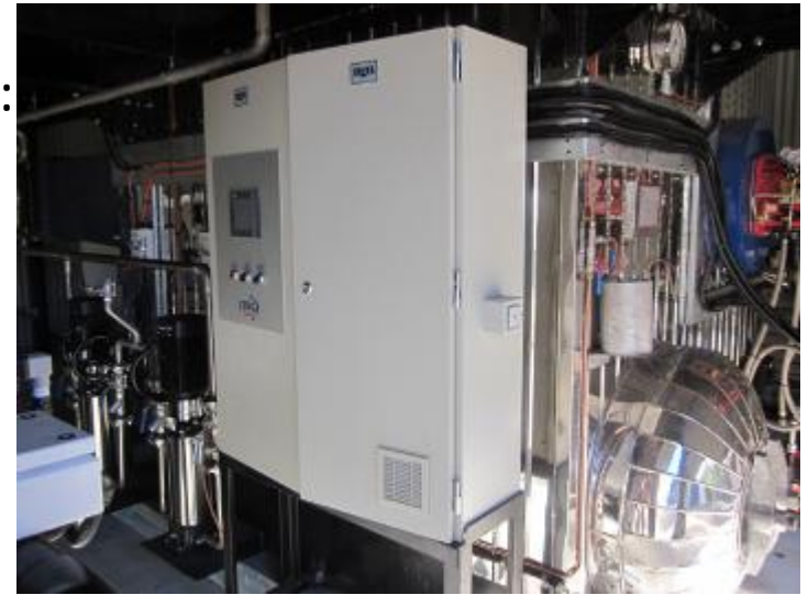
Boiler control panel
