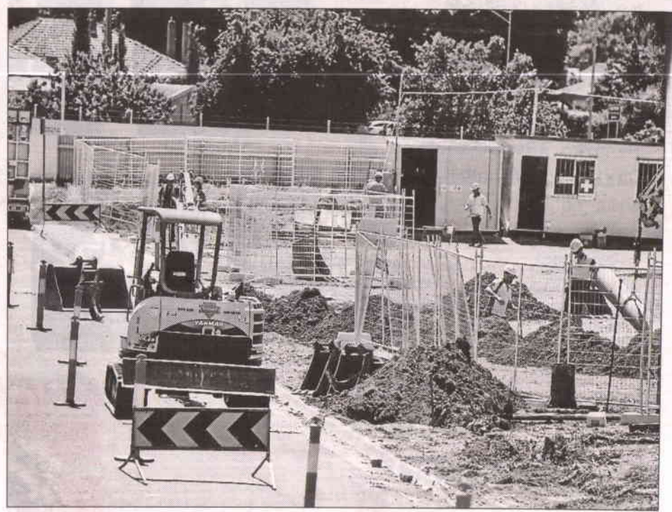
CONSTRUCTION ZONE: Work starts on the new ambulance station in Uley Street.
